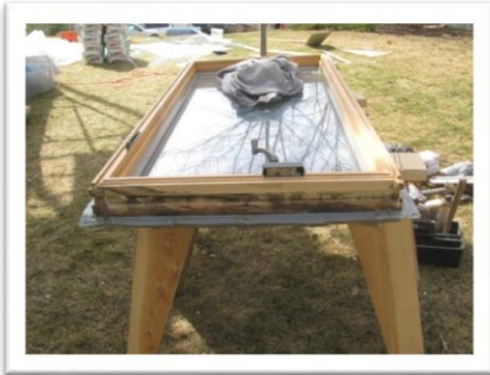
Damaged window frame
