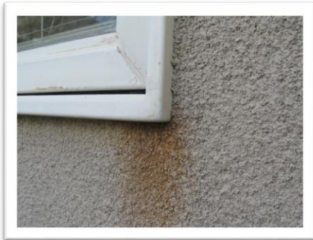
Discoloration. Water being directed out and over the stucco.
