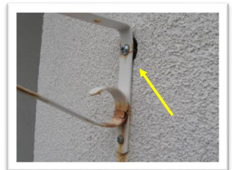
Penetration is not sealed
