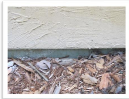
Stucco is terminated above grade
