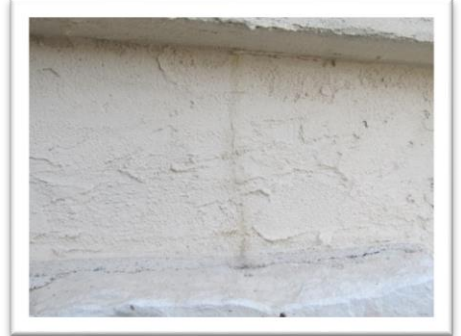
Crack with efflorescence
