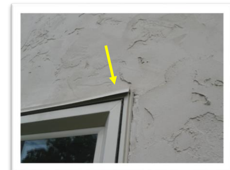
Flashing is too short, doesn't cover entire window and has negative slope.
