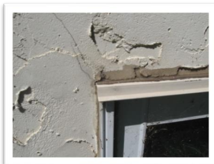
Caulking over head flashing - improper
