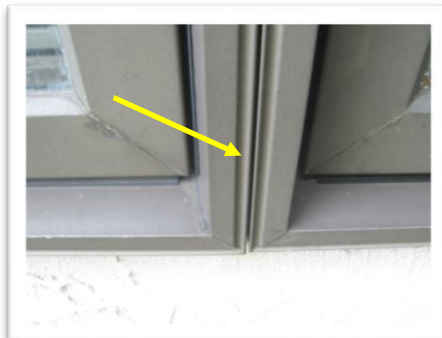
Window mullion joint, not capped
