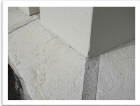
Column is not flashed or caulked
