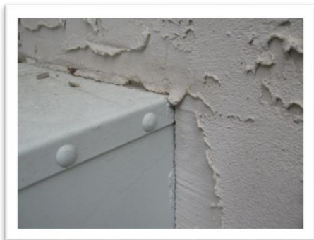
Utility is embedded and is not flashed or caulked
