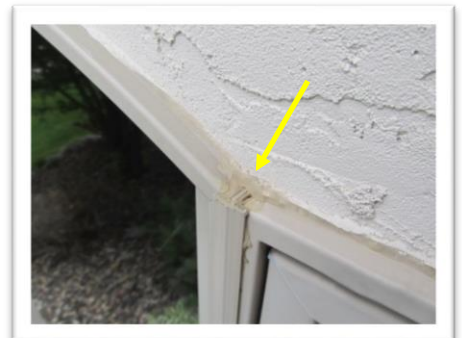
Vertical window mullion joint not flashed
