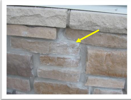
Efflorescence on stone application
