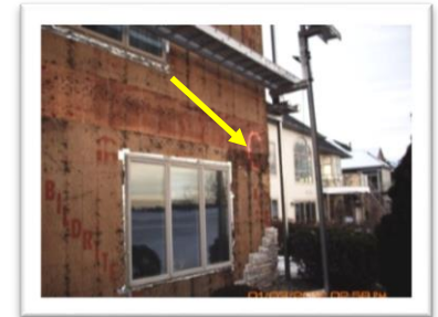
Rim joist damage from interior condensation
