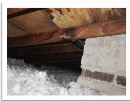
Attic/roof damage below ice damming
