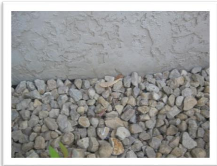
Stucco terminated below grade
