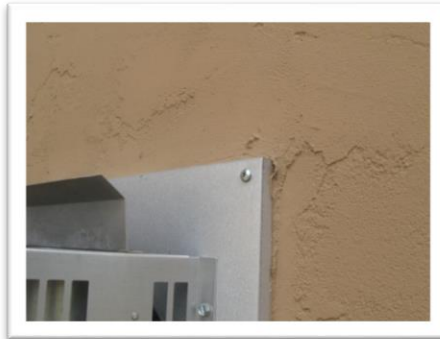
Fire flue is not flashed or caulked
