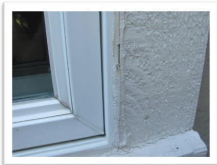
Caulk at window adhesively failing and needs maintenance
