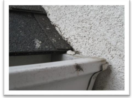
No kickout flashing present
