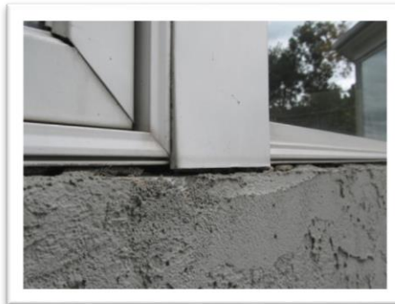
Window/stucco joint is not sealed
