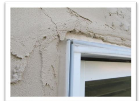
Good caulk joint, but behind the stucco, not over the stucco.
