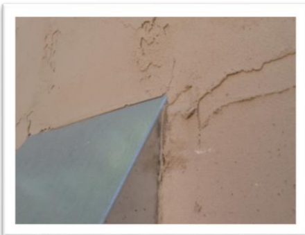
Vent is not caulked
