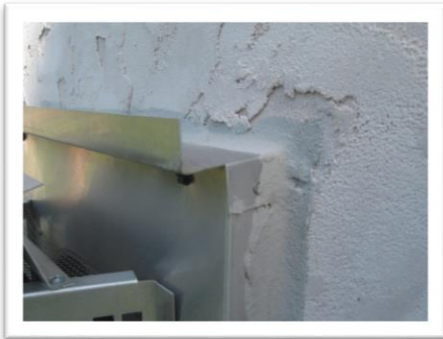
Fire flue is caulked
