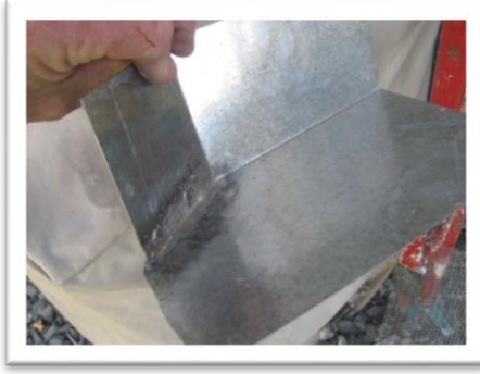
Kickout flashing with welded joints. Good
