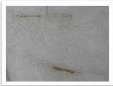
Cracks with staining. Water is behind the stucco.
