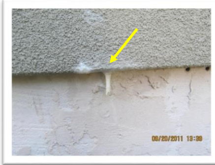
Efflorescence on stucco
