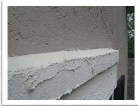
Accent is sloped away from the home
