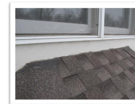
Dormer flashing missing
