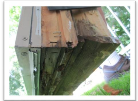
Damaged window frame
