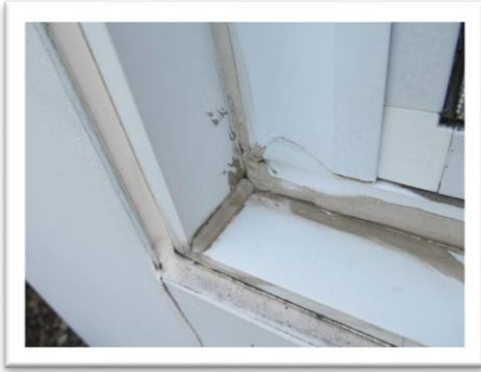
Poor caulk joint at a window joint - Adhesively failing
