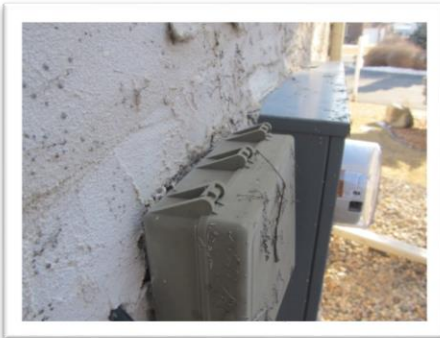
Utilities not flashed or caulked
