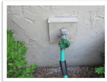
Hose bib is flashed
