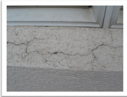
Accent is cracked with stains
