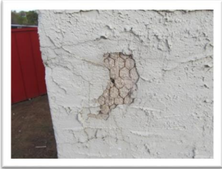
California one-coat stucco - spalling
