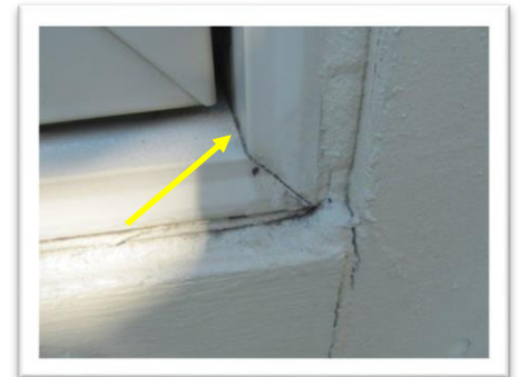
Window mitre joint is not sealed
