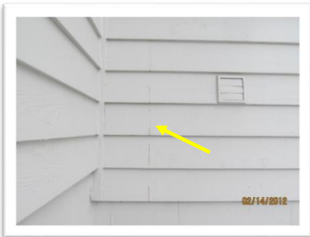
Stains over wood
