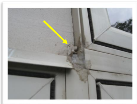
Caulk being used in a high risk area. Not a good application for caulk
