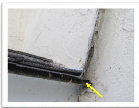
Improper kickout flashing installed on top of the step flashing.
