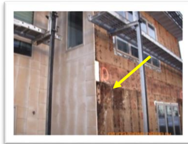
Rim joist damage from interior condensation
