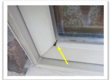
Sash with open corner, needs maintenance.
