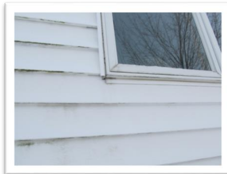
Stains over vinyl
