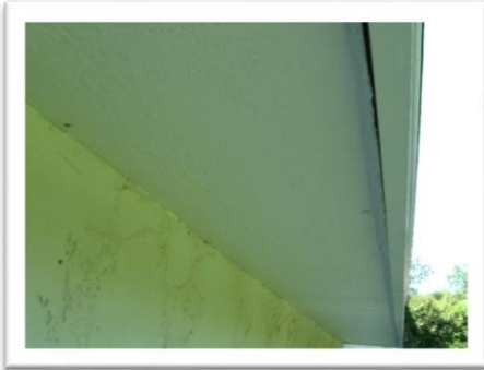
No ventilation through the soffit
